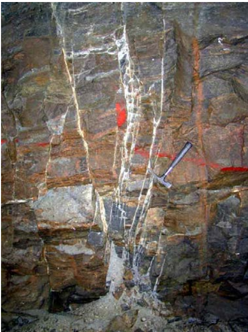
Figure 4: A small coarse fragmented weakness zone in a tunnel wall. White traces are filling of clay material.
